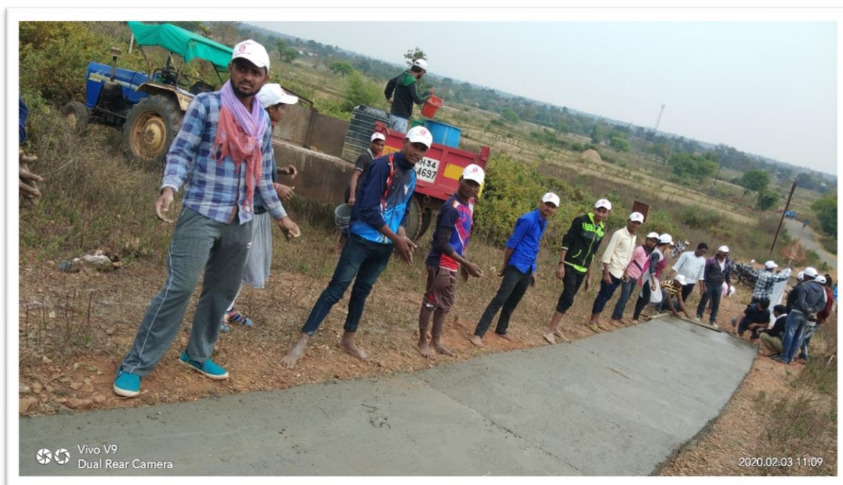
The NSS volunteers giving the final touch to the work of the construction of the cement-concrete ramp.
