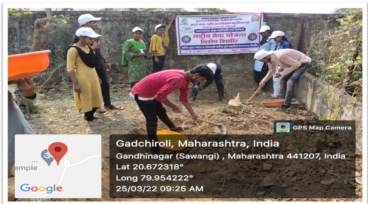
Students Digging the pit for making compost from waste generated by the school at adopted village under labour donation camp
