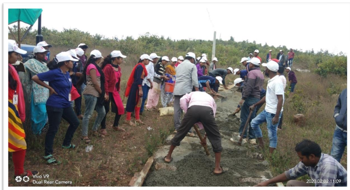
The NSS volunteers and villagers at the work of the construction of the cement-concrete ramp.
