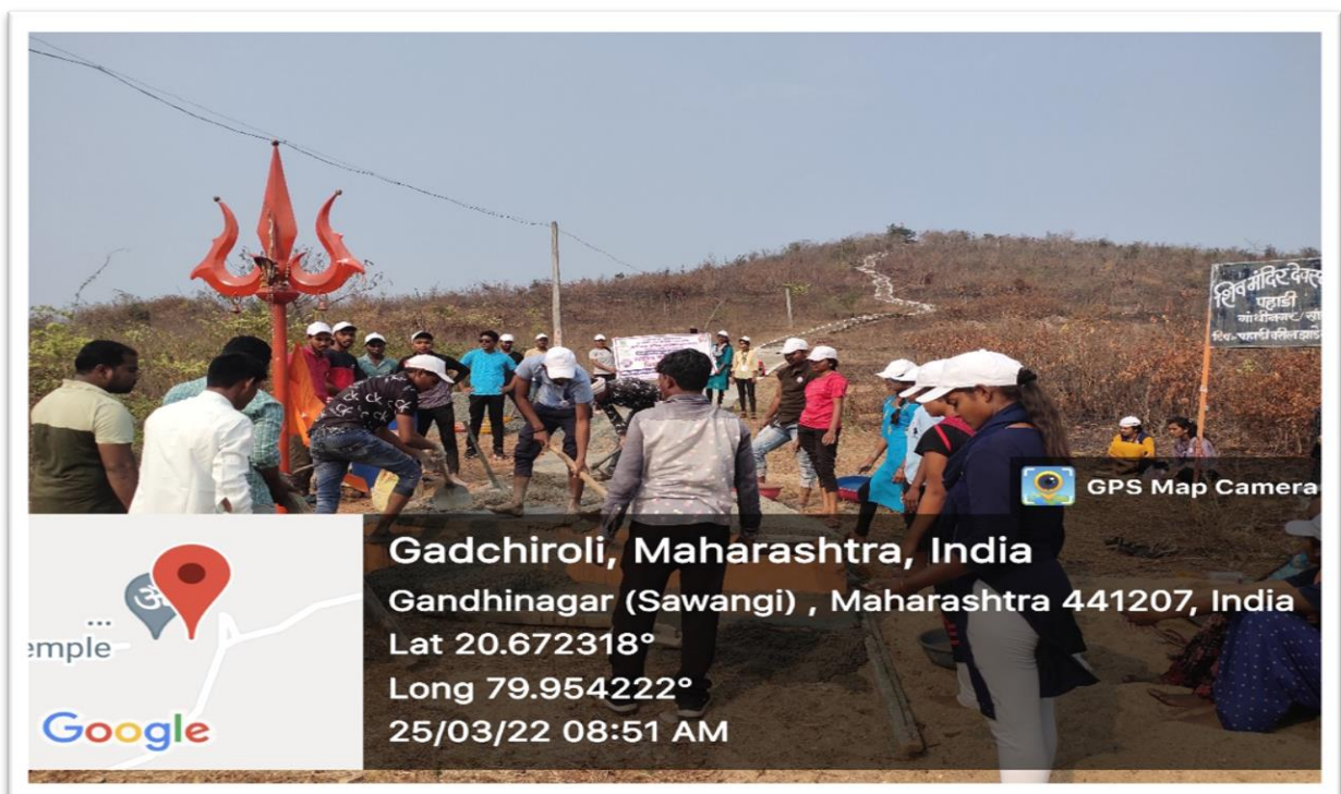
Through labour donation Students constructing the Ramp on the hill to walk to shiv temple
