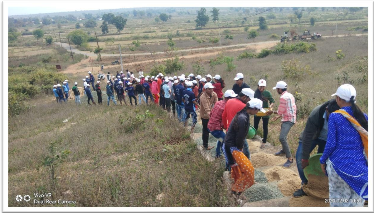
The NSS volunteers and villagers at the work of the construction of the cement-concrete ramp.
